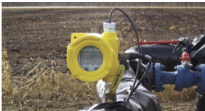
Typical DCR1000 installation
